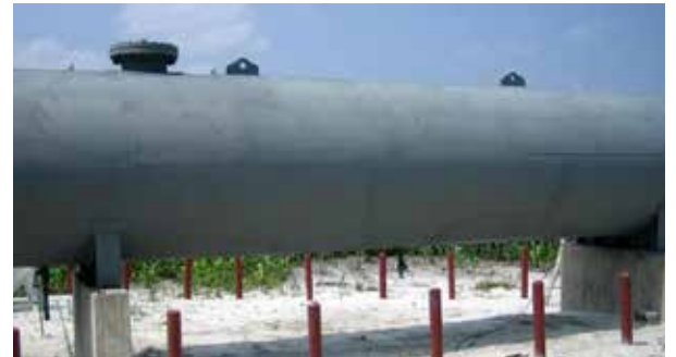
Vessel coated with Belzona 6111 providing a cathodic protection to the metal surface
